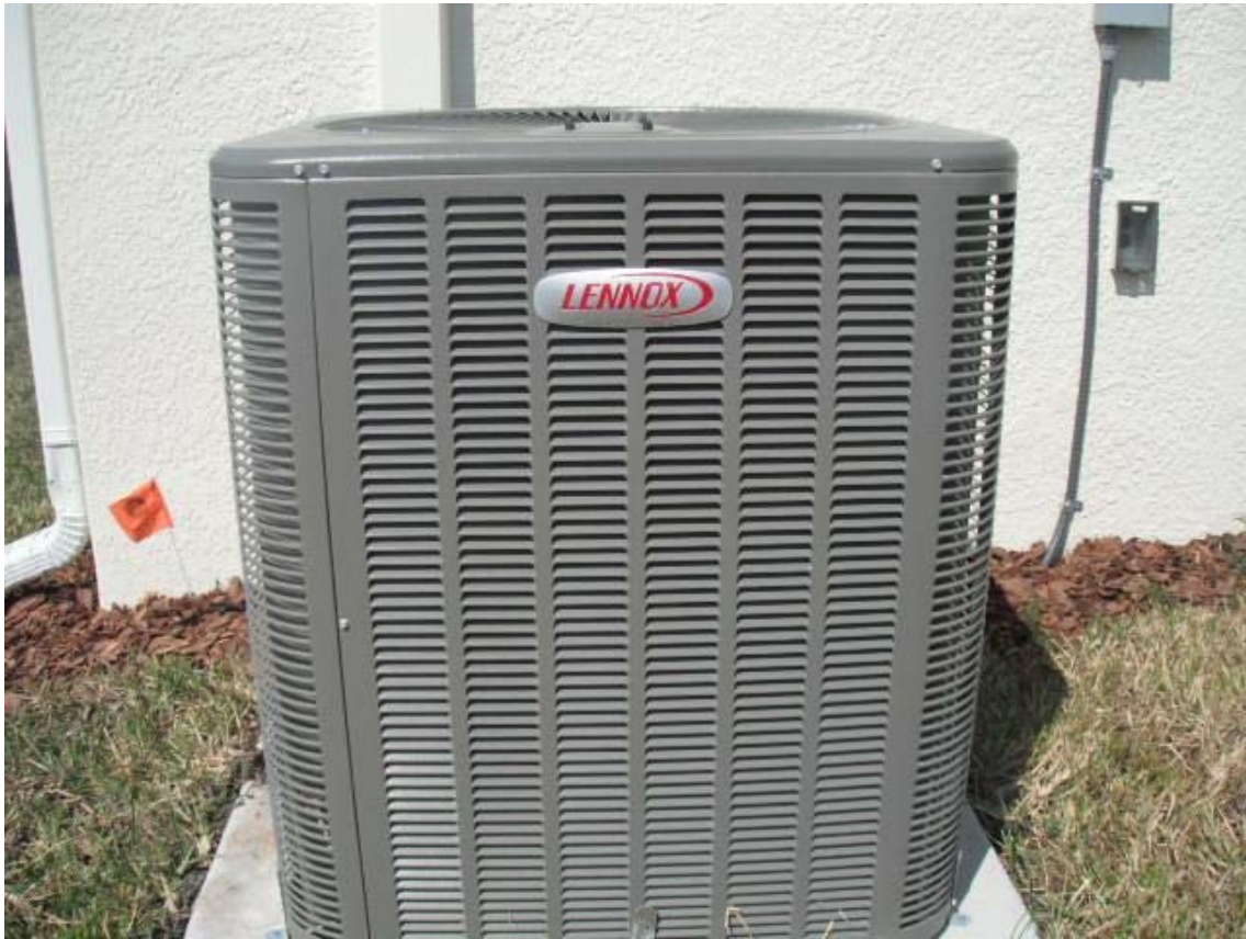
AC Condenser - Working
