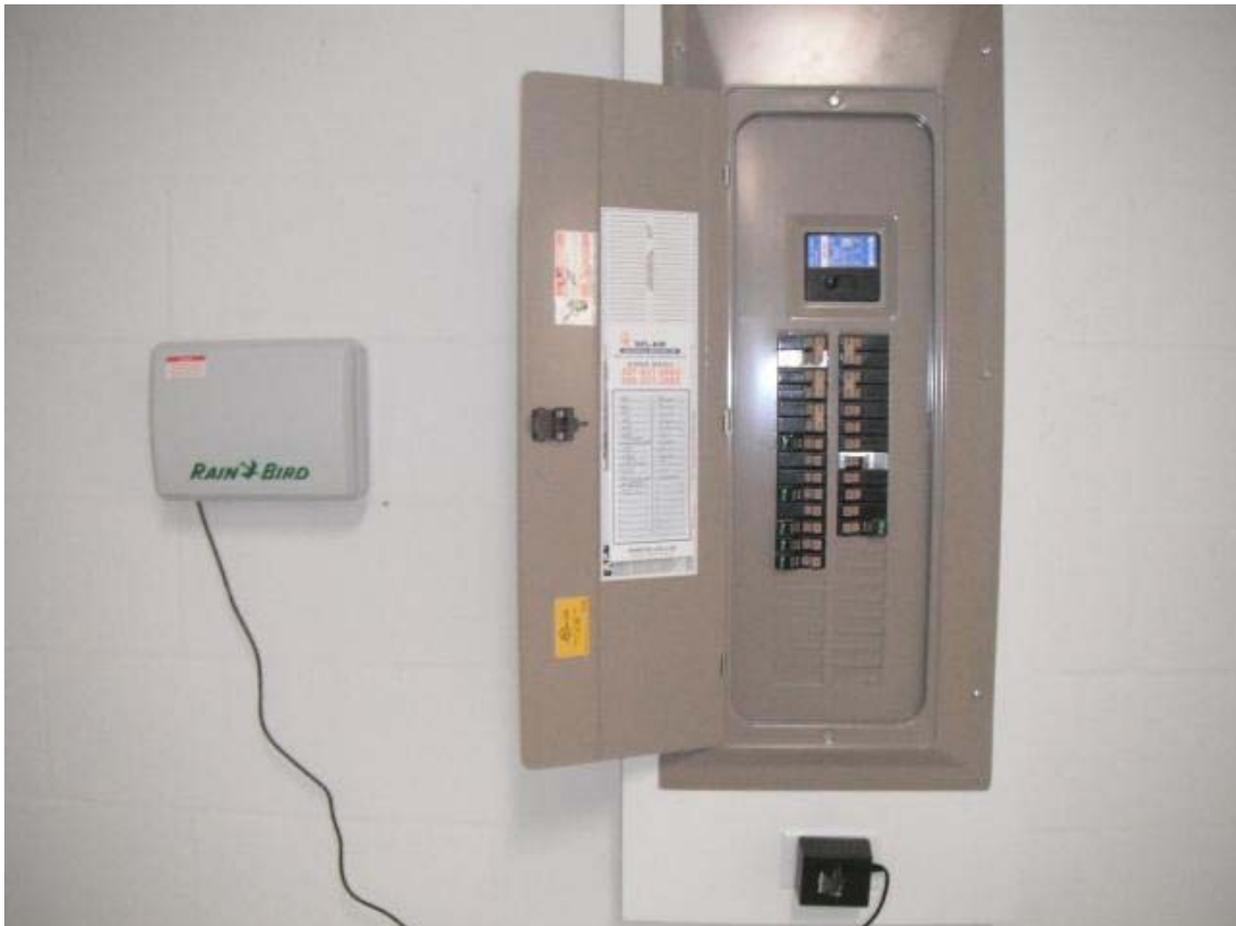
Main Electric Panel
